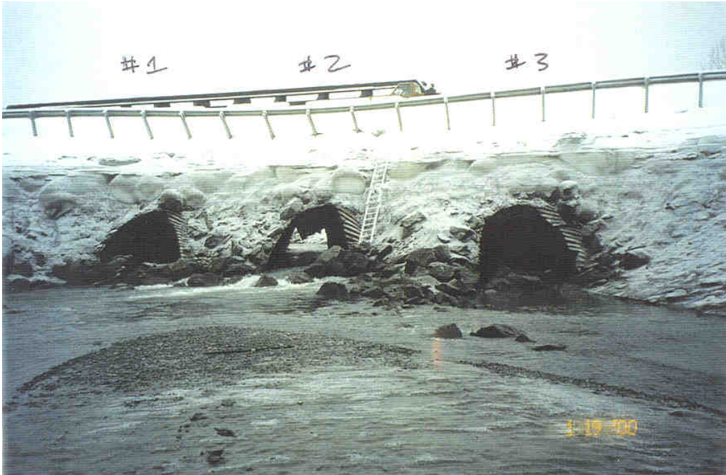
Photo 1: Downstream side of three existing culverts and embankment failure.
