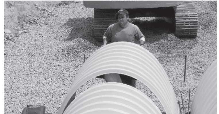
Continue installing chambers by overlapping chamber end corrugations. Chamber joints are labeled "Lower Joint – Overlap Here" and "Build this direction – Upper Joint". Be sure that the chamber placement does not exceed the reach of the construction equipment used to place the stone. Maintain minimum 9" (300 mm) spacing between rows. For the Isolator Row place two continuous layers of ADS Woven fabric between the foundation stone and the isolator row chambers, making sure the fabric lays flat and extends the entire width of the chamber feet.
