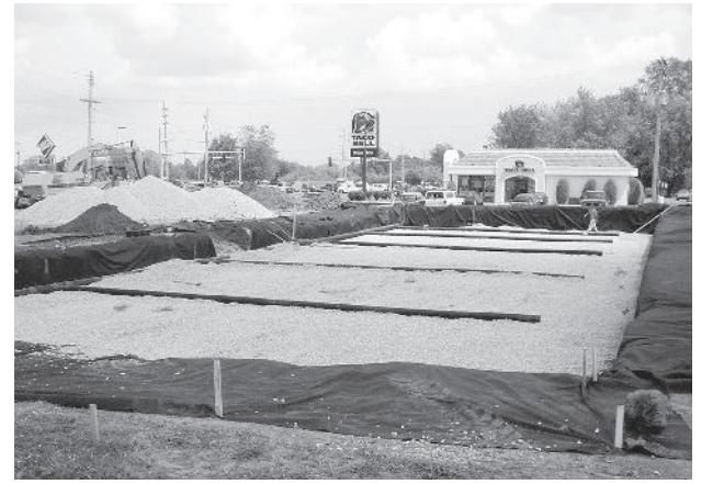
Place clean, crushed, angular stone foundation 9" (230 mm) min. Install underdrains if required. Compact to achieve a flat surface.
