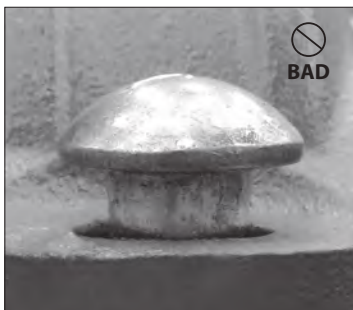
BAD BOLT ENGAGEMENT (OVAL NECK IS NOT SEATED PROPERLY IN THE BOLT HOLE)
