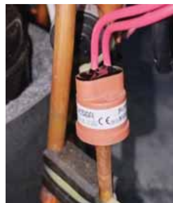
High Pressure Switch
