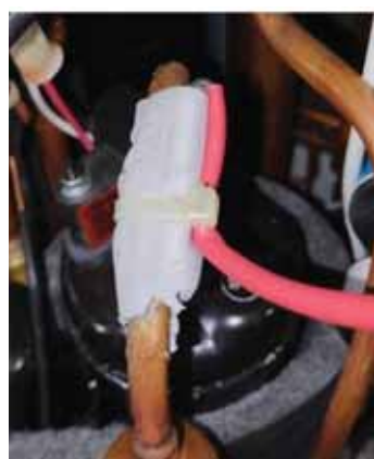
Discharge Temperature Sensor
