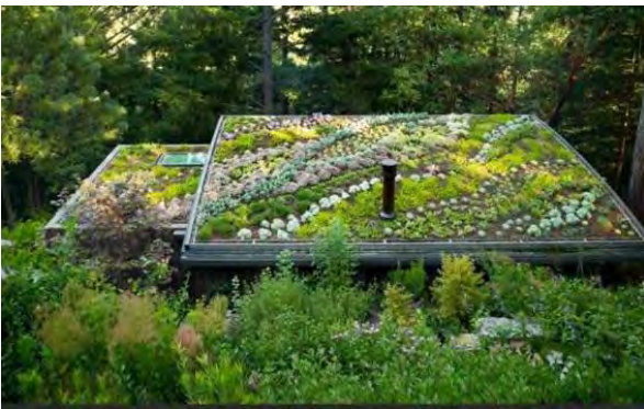
Vegetated roof slows stormwater runoff.
