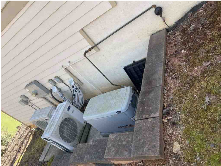
Mini-Split A/C units & whole home generator
