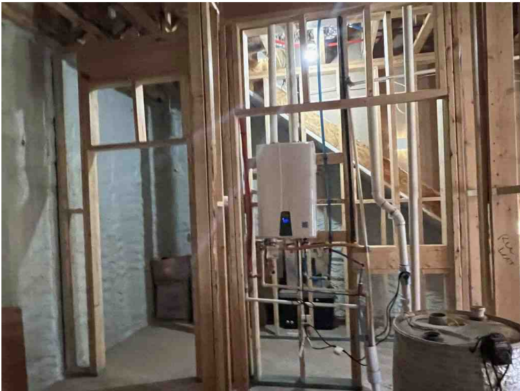
Unfinished basement - tankless water heater
